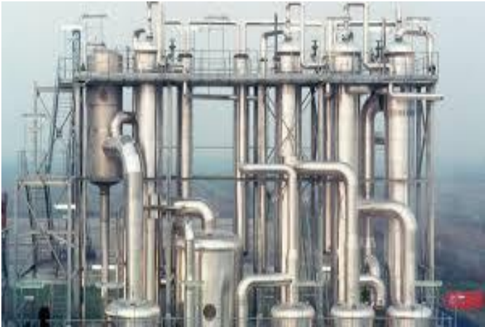
Zero Liquid Discharge Plant
