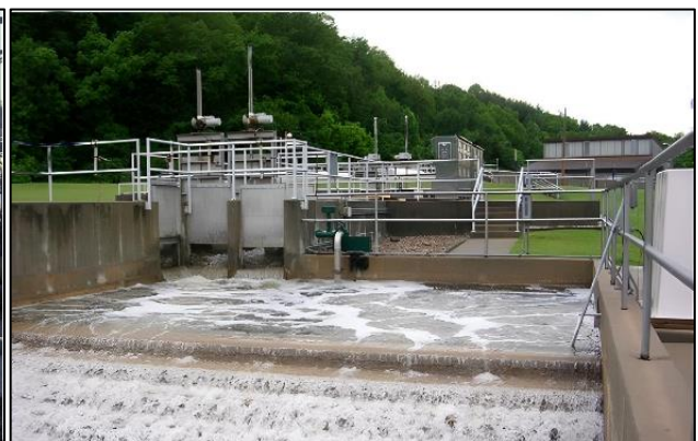
Sewage Collection Tank & Cascade Aerator
